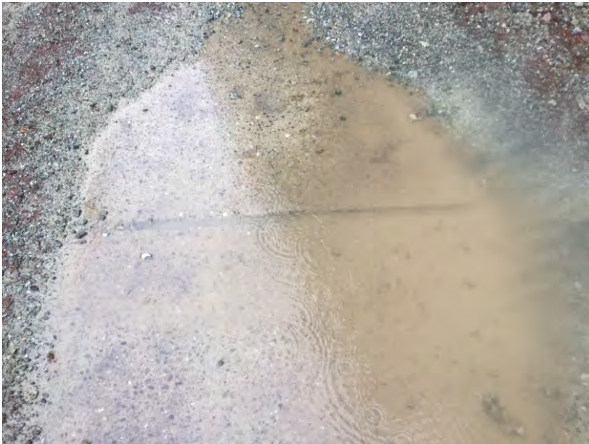
Grout on deck joints not flush with deck
