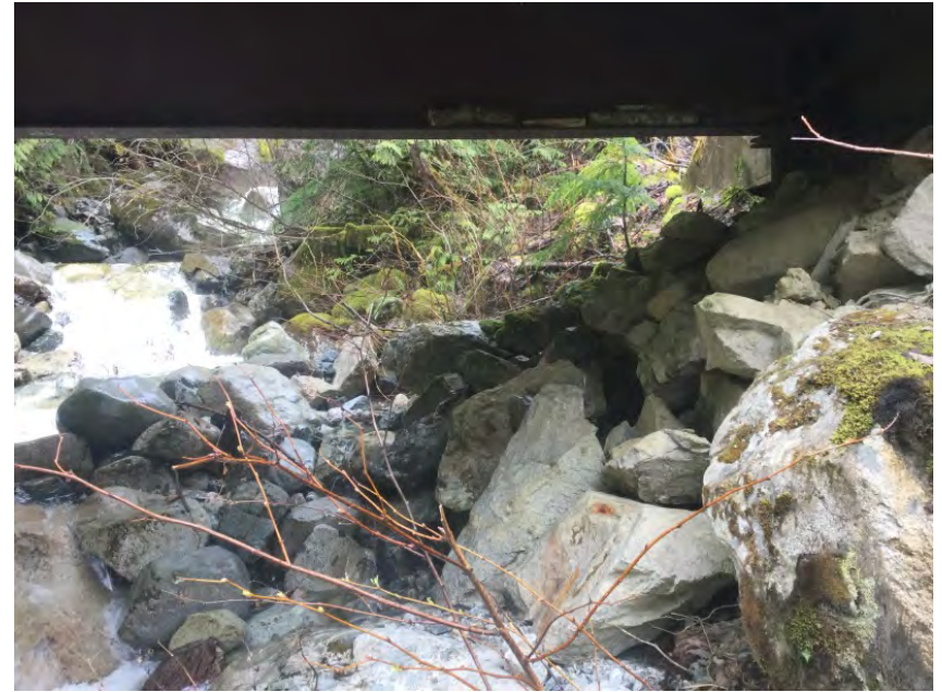
Riprap at left bank scour
