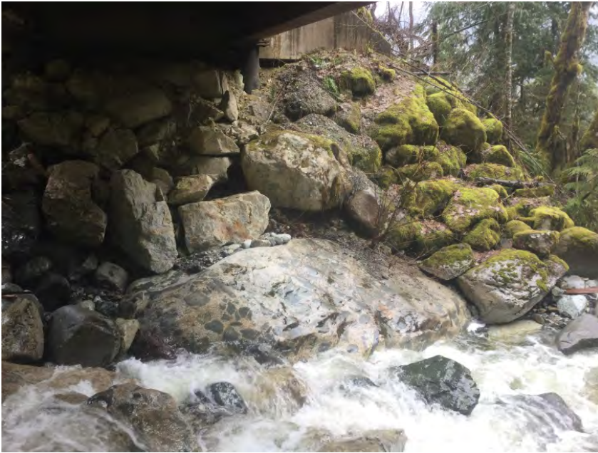
Riprap at left bank has been undermined and starting to shift
